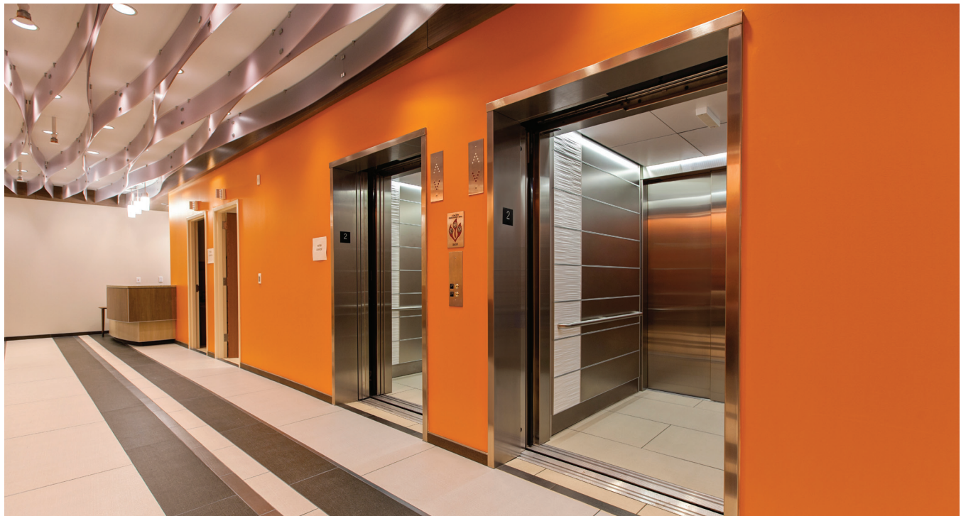
LEVELe-103 Elevator Interiors with panels in Stainless Steel with Seastone finish, and Bonded Quartz, White, with Kalahari pattern
